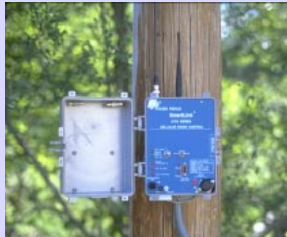
Series 2700 SmartLink Fault Monitor and Control Unit Pole Mounted within 100' of Field Reporting Units
